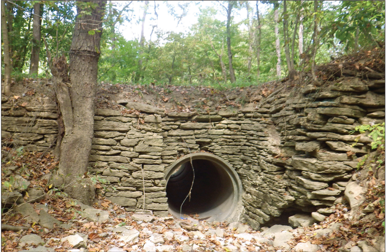
Figure 4.2 Stacked limestone retaining wall and culvert along KY2885, 40 meters west of its intersection with Netherton Lane.
